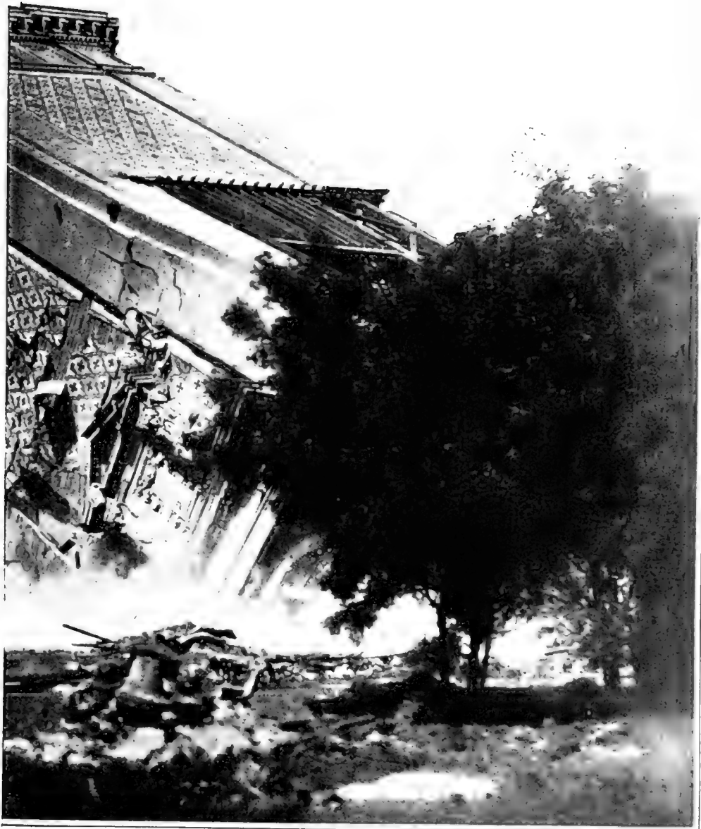
was dynamited and the big pillar crashed to earth, a mass of splintered wood
